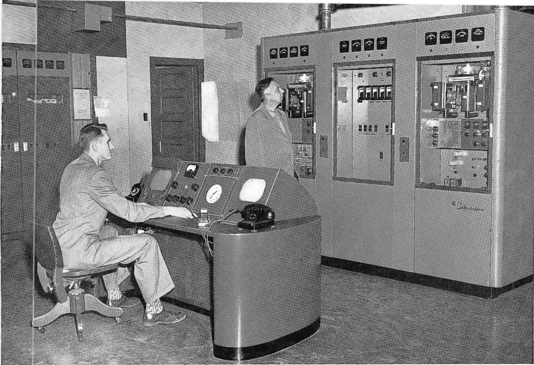
FIG. 2. Main room of TV transmitter building. Charles Sakoski, Sr., Chief Engineer, checks 1 KW RCA UHF transmitter, while Joe Emashowski, Jr. operates console. In the rear is 1 KW RCA FM transmitter. Room through door in rear is workshop and store-room.
